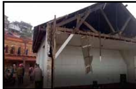
An image revealing the demolition of the monastery. Photo credit: Kalsang Norbu
